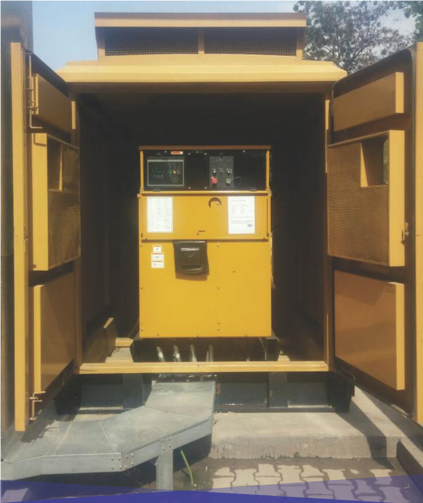
PTCL POWER HOUSE SATELLITE TOWN RAWALPINDI.
