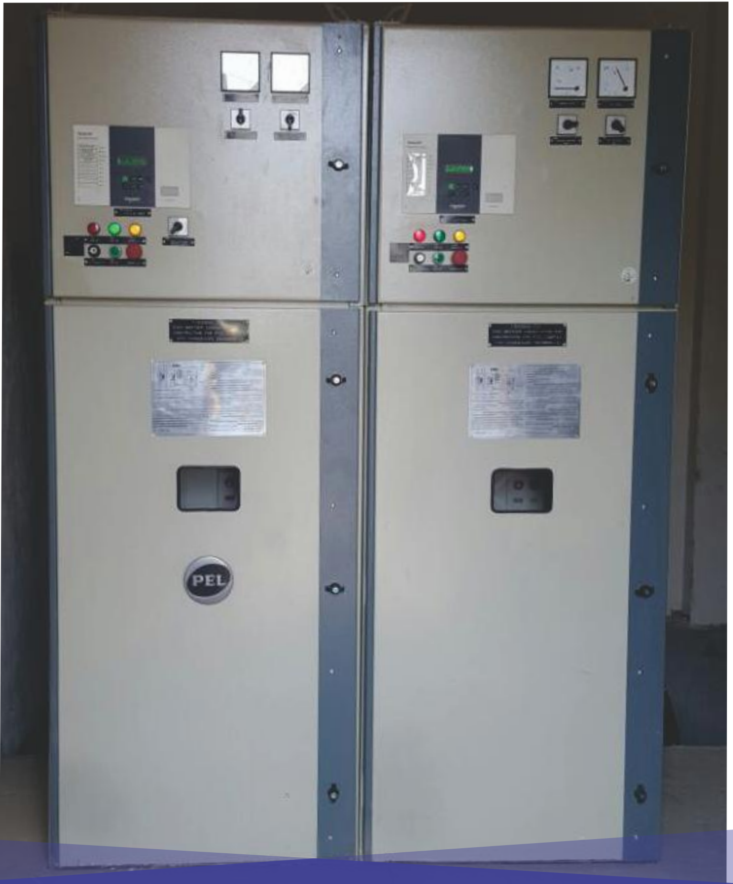
PTCL POWER HOUSE SATELLITE TOWN RAWALPINDI.
